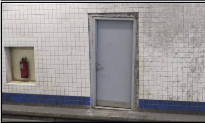
What's wrong with this picture? (The door is level—the doorframe parallels the roadway, which is inclined toward the tunnel exit.)
